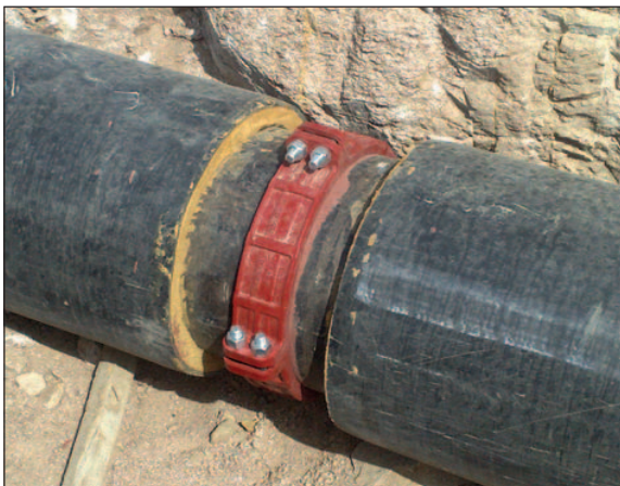
A 700mm (28") R-88 coupling installed in a chill water system
